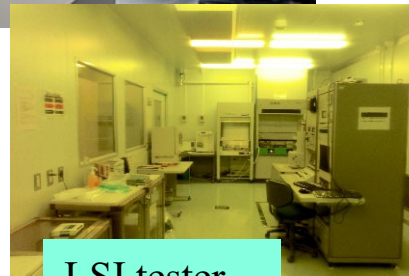
LSI tester Clean room
